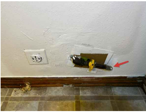
Kitchen- Gas Pipe
