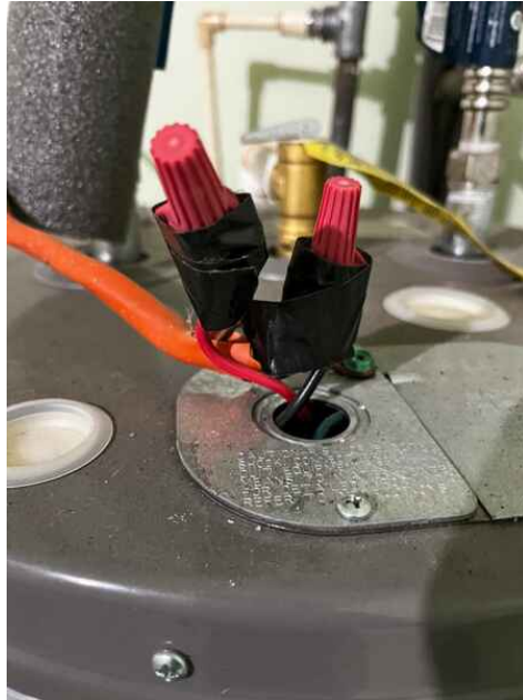
Garage- Water Heater
