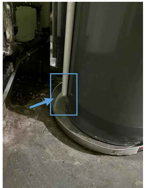
Garage- Water Heater TPR Valve
