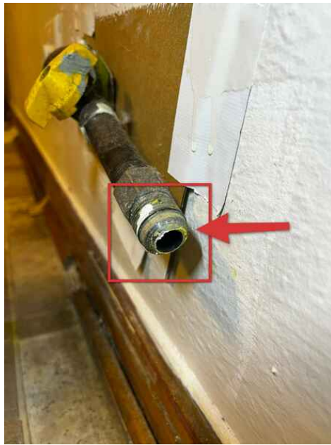
Kitchen- Gas Pipe
