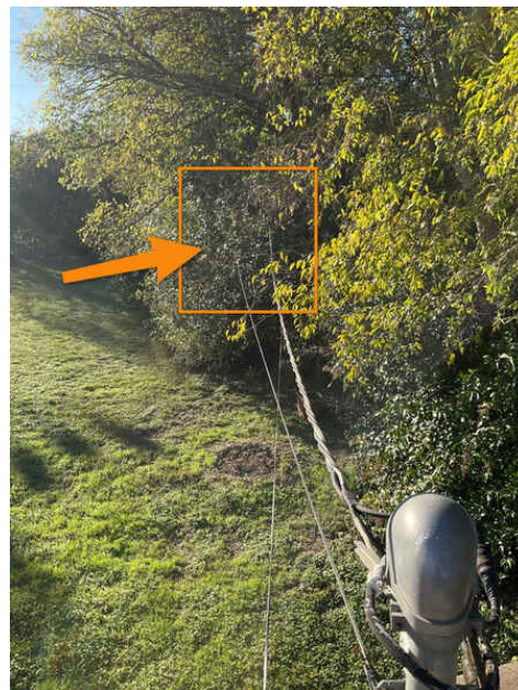
Overhead Mast Wiring
