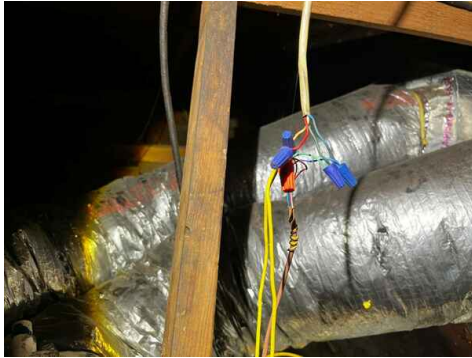
Attic- HVAC Unit
