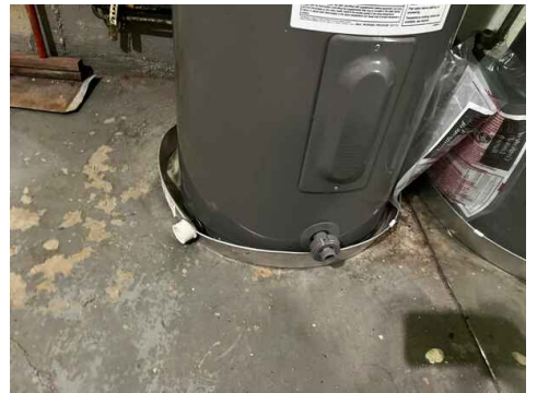
Garage- Water Heater Overflow Pan Discharge
