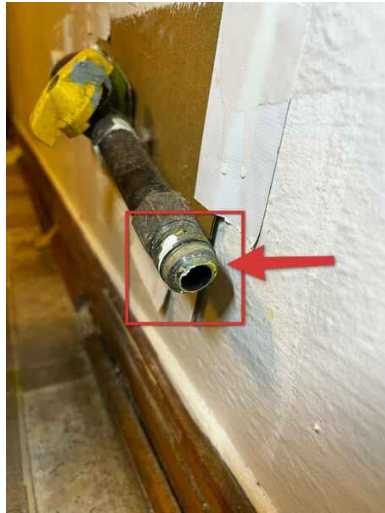
Kitchen- Gas Pipe
