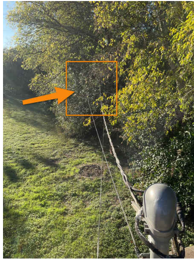
Overhead Mast Wiring
