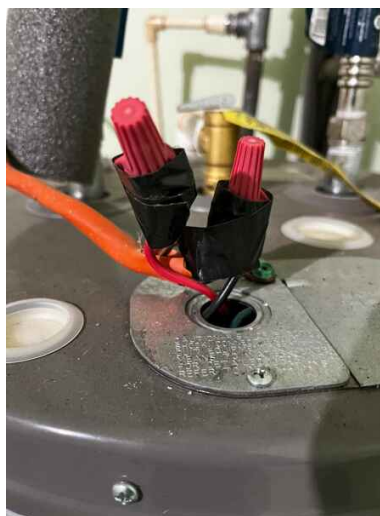
Garage- Water Heater
