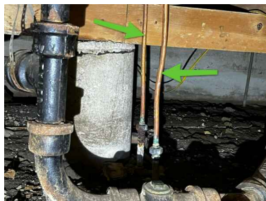
Crawlspace- Water Distribution Pipe
