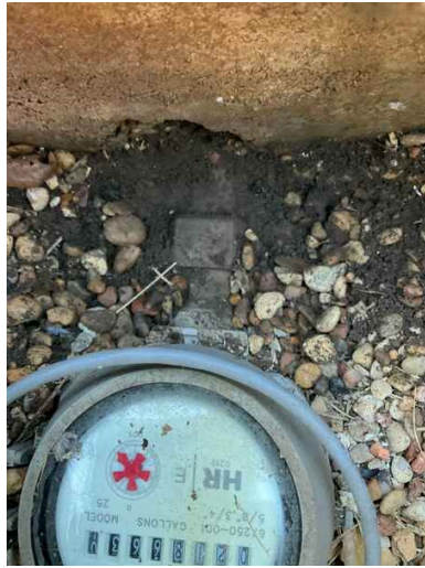
East- Water Meter
