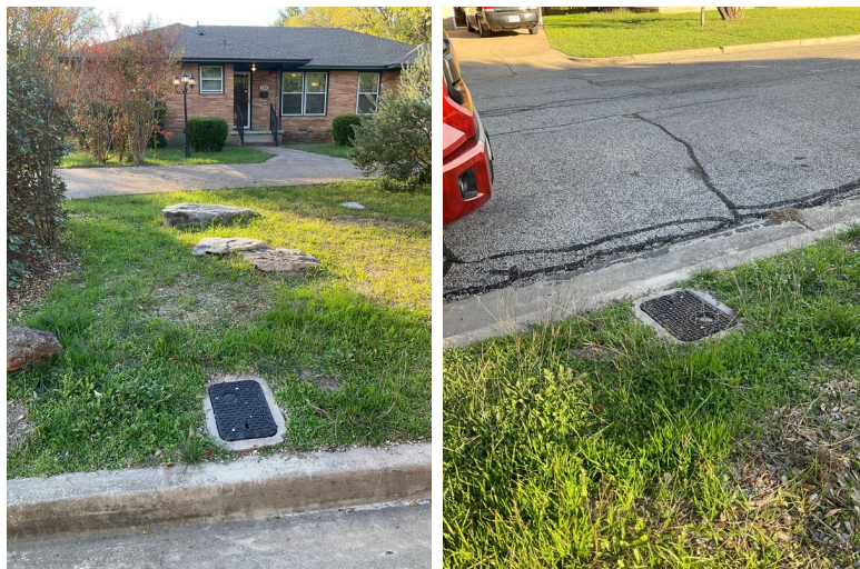
Location of Water Meter: Exterior
