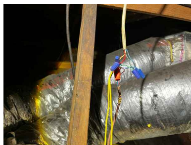
Attic- HVAC Unit
