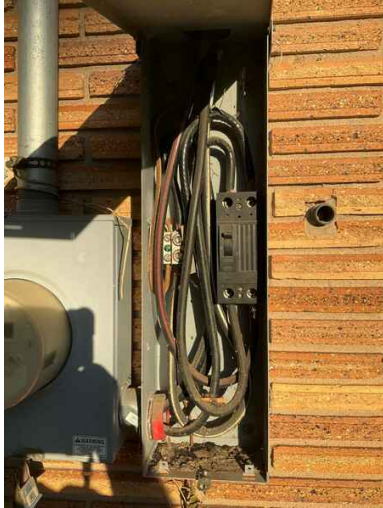
Main Service Panel Breakers
