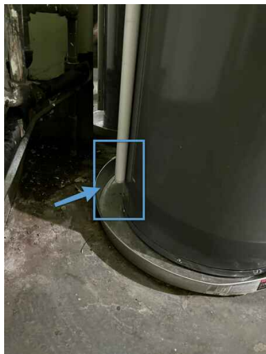
Garage- Water Heater TPR Valve
