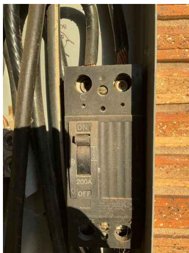
200 AMP Main Breaker
