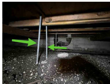
Crawlspace- Water Distribution Pipe
