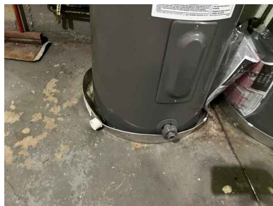
Garage- Water Heater Overflow Pan Discharge
